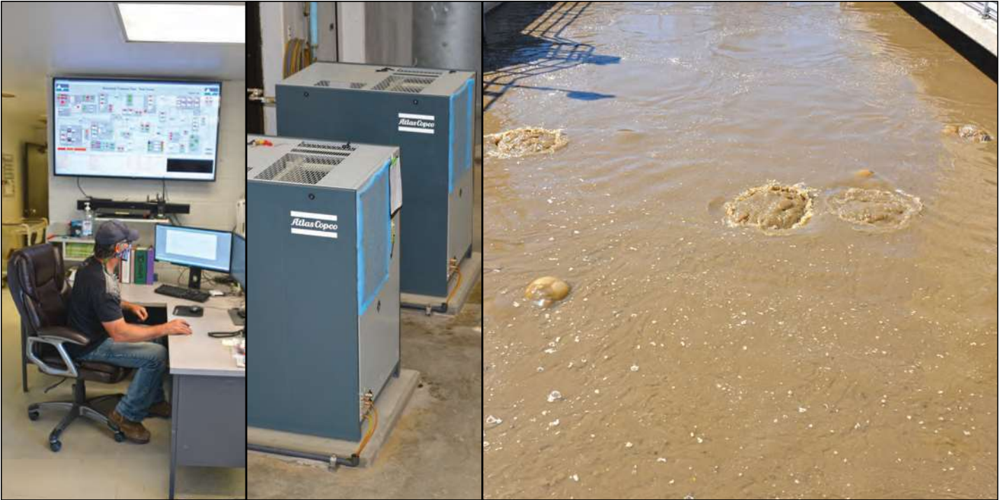
Joe Creaghe sits at the SCADA workstation, at the Loveland Water Reclamation Facility, preparing to tell the system what tanks to create bubbles in, when to create them, and for how long to release the air.
