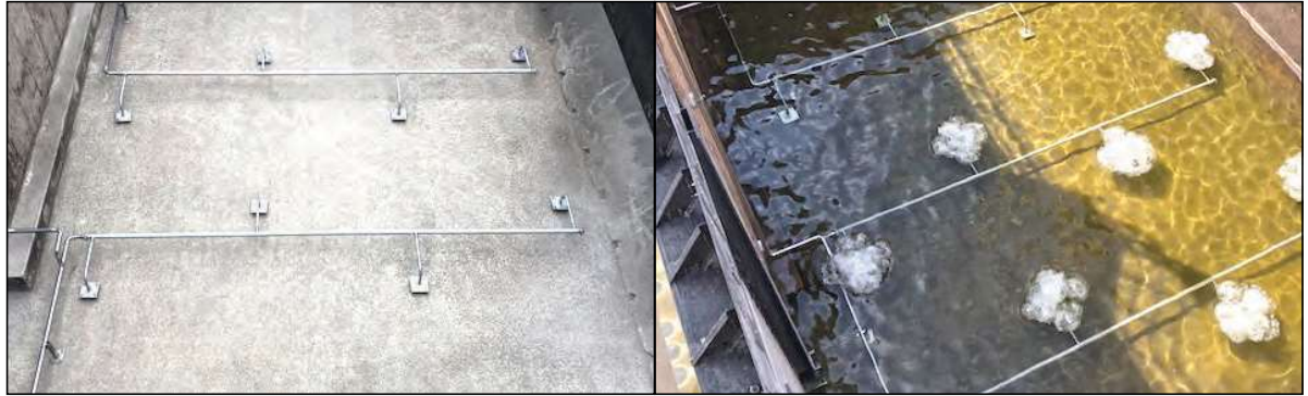
Pipes and nozzles installed in the tank before (left) and after water is added.
