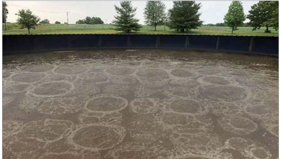
Shown is the new aerobic digester at the City of Highland's HWRP.
