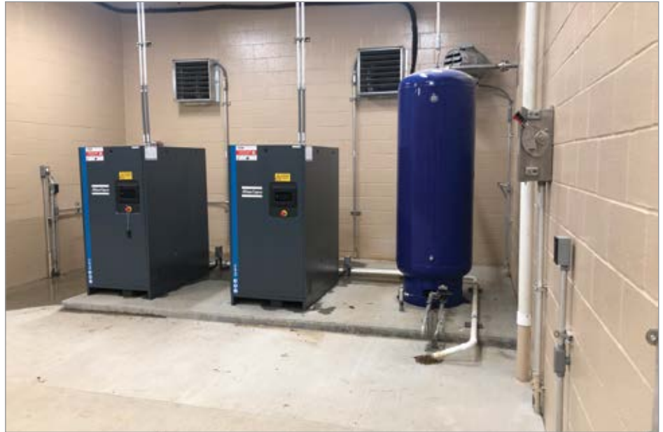
Air compressors provide high-pressure air for the compressed gas mixing system at the City of Highland's HWRF.
