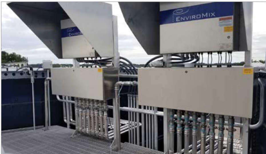
Figure 5: Local control panels distribute the optimal mixing energy.
