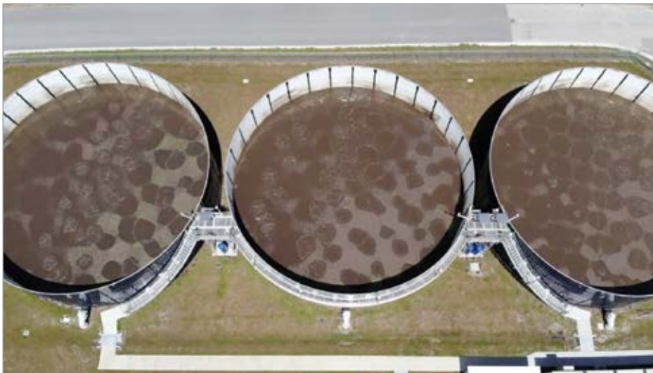
Figure 3: Short-duration bursts of compressed air mix an area of the tank 2-3 times per minute.
