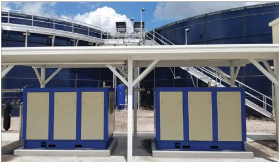
Figure 4: Compressors under a canopy meet the process mixing air demands of the BioMix system for all three equalization tanks.
