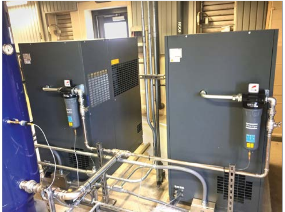
Figure 6: Low-maintenance compressor system matches mixing air demand with duty and standby configuration.
