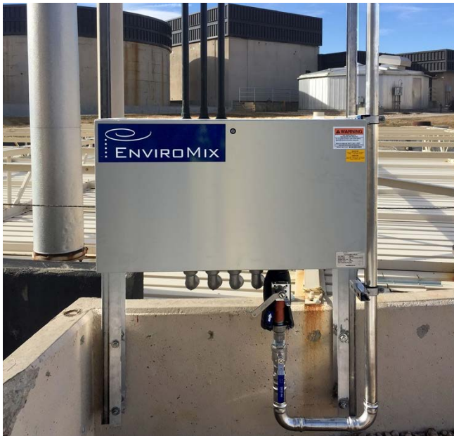
The valve control module enables the optimal mixing regime by controlling air release duration, frequency, and sequence.
