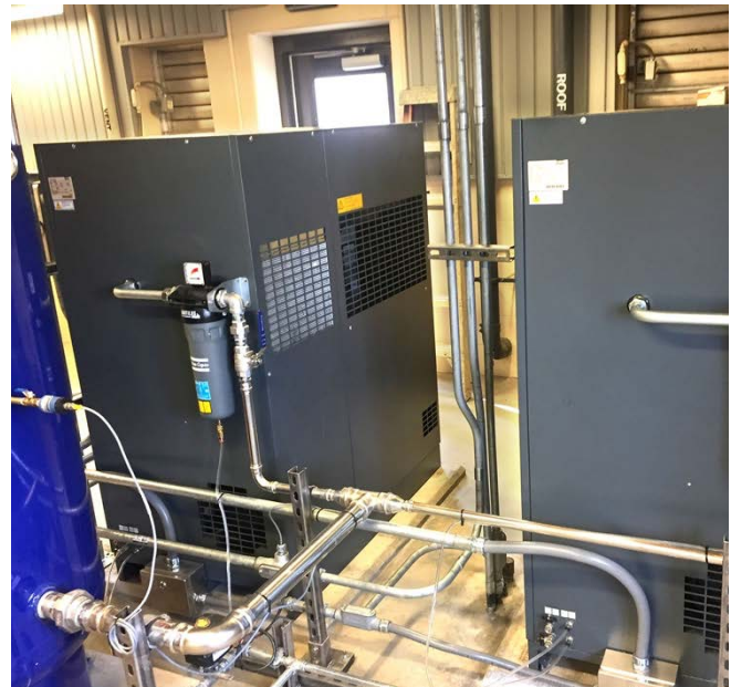
Low maintenance compressor system matches mixing air demand with duty and standby configuration.
