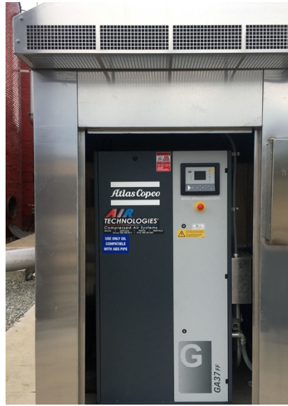
Compressor is housed in an environmental enclosure to eliminate the need to construct a building
