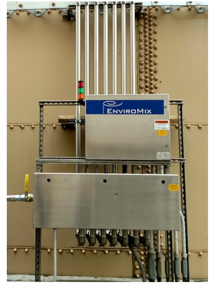
EnviroMix control modules allow for adjustable mixing intensity to match system demands
