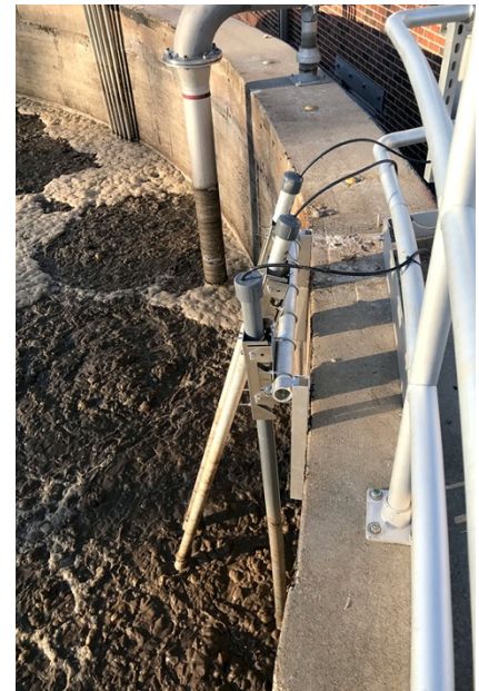
Level, DO, and ORP instrumentation
