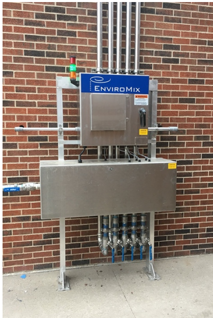
Valve control module located at the digester controls the mixing intensity
