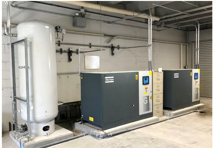
Compressors and receiver are located indoors for ease of maintenance
