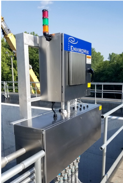
BioMix is controlled and monitored from an easily accessible control panel
