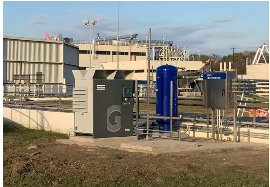
Compressor, receiver tank, and valve control panel deliver high pressure mixing air to the system with flexibility to optimize mixing
