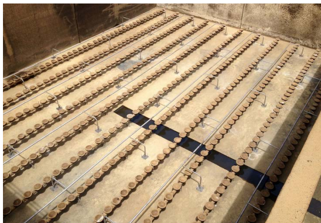
Aeration satisfies oxygen demand while BioMix compressed gas mixing maintains mixed liquor suspension
