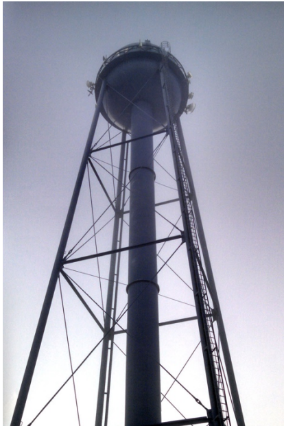
The elevated water storage tank at the Montana Law Enforcement Academy in Helena, MT.
