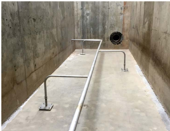
Nozzle headers are well-suited for long narrow basins.
