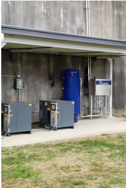
The Zombie valve control module optimally controls mixing regime through operator adjustable settings for duration and frequency of nozzle firing
