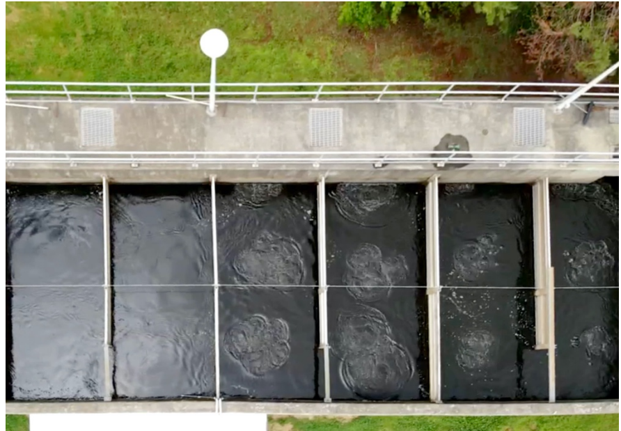
The serpentine flow pattern of the PAC contactor would have required eight mechanical mixers versus two scroll compressors (one duty, one standby)
