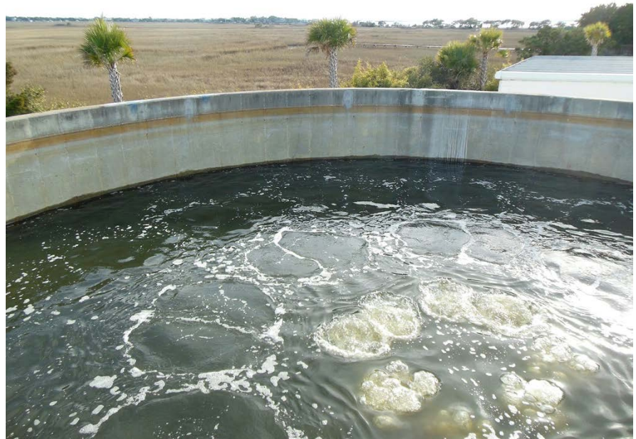
Short duration, sequential bursts of compressed air uniformly mix the tank contents.
