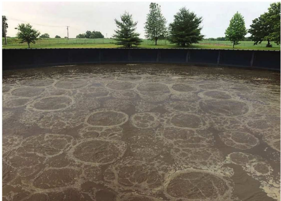
Figure 8. The new aerobic digester at the City of Highland's HWRf.
