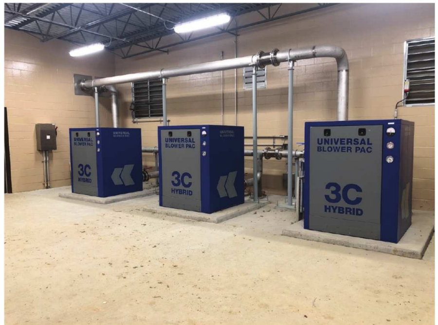
Figure 2. EnviroMix's modified approach to aerobic digestion can use hybrid rotary screw blowers to provide efficient aeration, in turn, satisfying oxygen demand for VS destruction.
