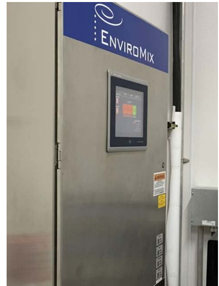
Master Control Panel (MCP) allows operators to control firing parameters from a climate-controlled room.
