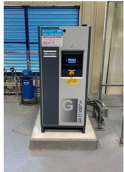
Duty and standby compressors charge the receiver tank which supplies compressed air to the valve module.
