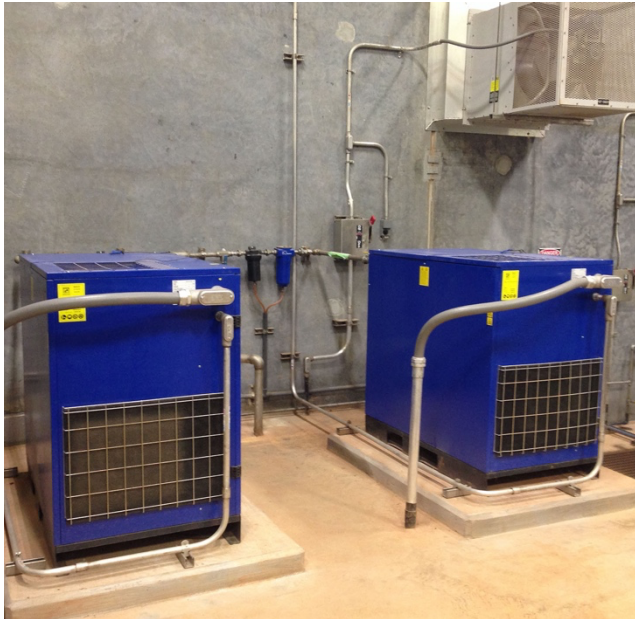
Compressed air is provided by duty and standby compressors
