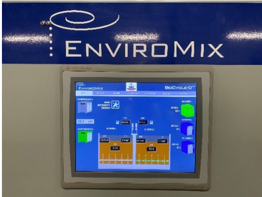
From the operator interface terminal (OIT), operations staff can monitor all equipment and control the aerobic digestion process.
