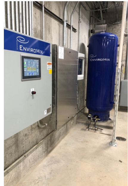
The Master Control Panel controls the BioMix system as well as the blowers through online instrumentation.
