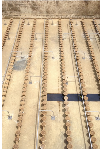
Decoupling aeration from mixing prevents over-aeration
