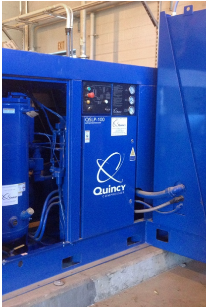
Two 100 HP compressors replaced dozens of mechanical mixers
