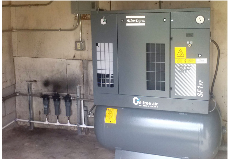
The easily accessible compressor in Opheim, MT.
