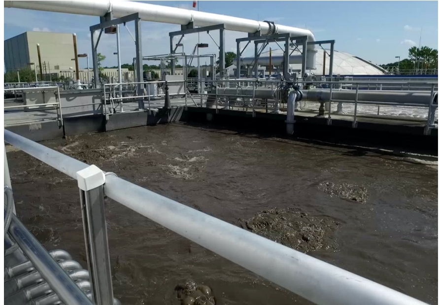
Short-duration bursts of compressed air fired intermittently produce optimal anoxic mixed conditions with a coefficient of MLSS variation of less than 2%.
