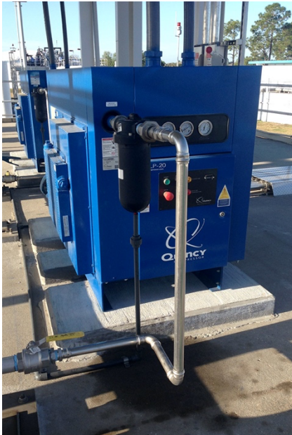
The BioMix system uses only one operating compressor as opposed to multiple mechanical mixers, significantly reducing maintenance for the City of Orlando.
