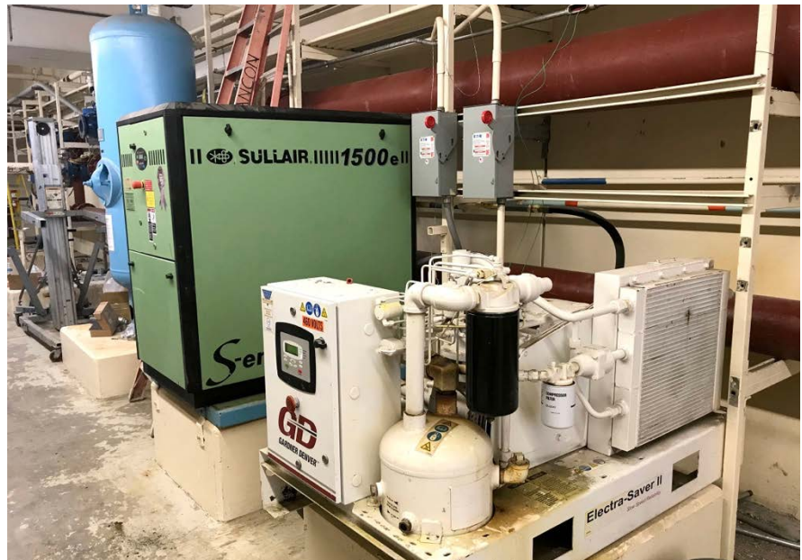
Existing compressor and receiver tank system that serves the BioMix system
