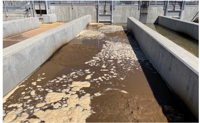
BioMix is used to continuously mix the anoxic selectors that follow the anaerobic selectors.
