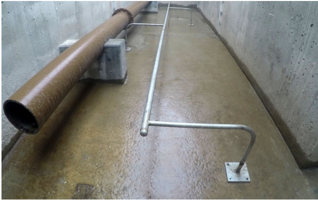
BioMix-DC nozzles provide gentle pulses of mixing energy to transport VFA from the fermentation layer to the PAOs throughout the anaerobic selector.
