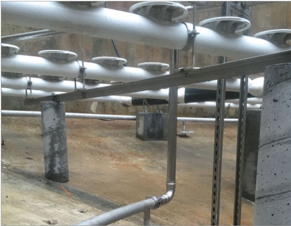
BioMix nozzles alleviate dead zones in the aerobic digester in Emporia, Kansas.
