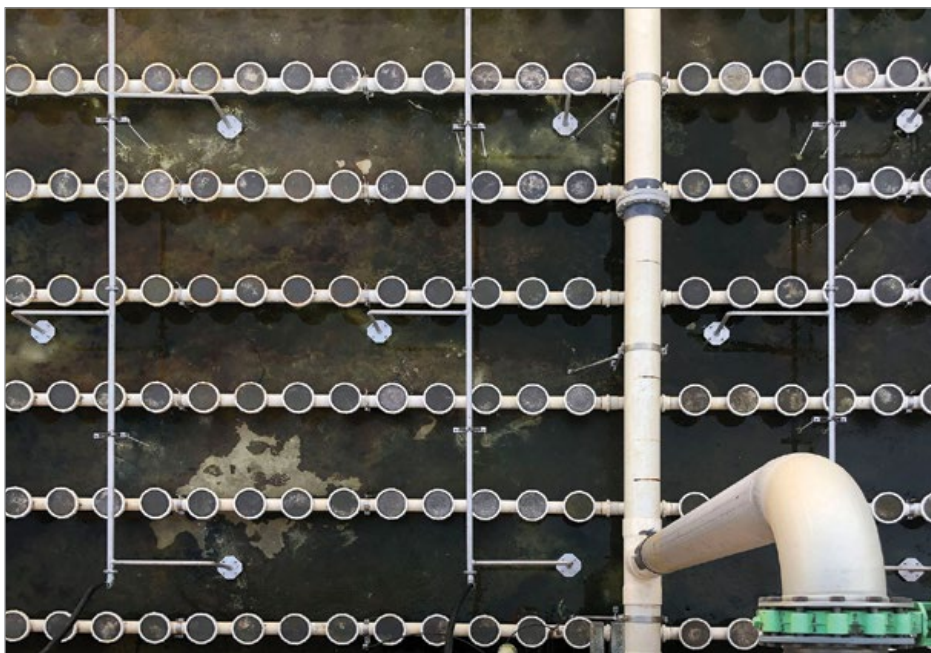
BioMix nozzles interlaced with diffused aeration.
