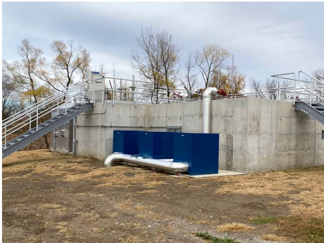
Positive displacement blowers provide low pressure air for the fine bubble diffused aeration system.
