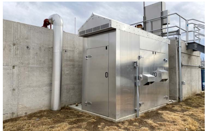
Rotary screw compressor housed in a weathertight ventilated enclosure provides high pressure air for the BioMix system.
