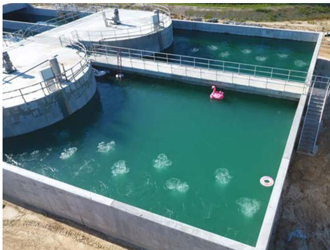
BioMix Compressed Gas Mixing System operating during startup of anoxic selectors.
