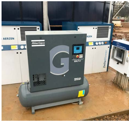
Blowers, compressor and master control panel located tankside
