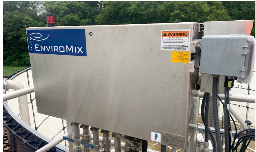
Zombie Valve Module located at top of tank
