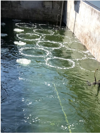
Installing the correct nozzle density is critical in the design of a compressed gas mixing system. Even with a partially full tank, an overlap in the zone of influence of each nozzle can be observed in the surface mixing pattern.
