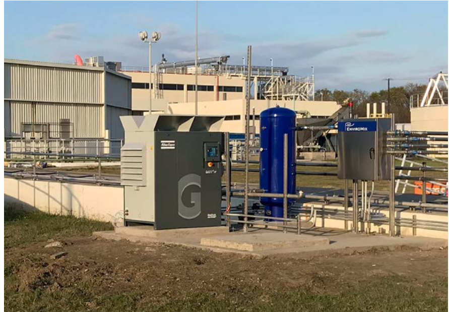
Compressor, receiver tank, and valve control panel deliver high pressure mixing air to the system with flexibility to optimize mixing
