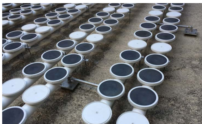
Nozzles seamlessly integrated with diffused aeration
