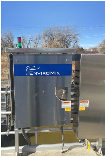
Custom control panels
