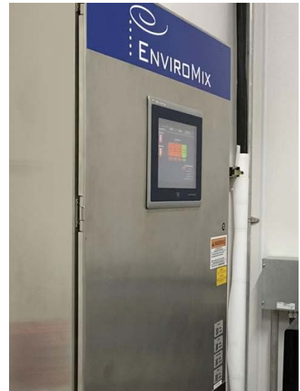
Master Control Panel (MCP) allows operators to control firing parameters from a climate-controlled room.
