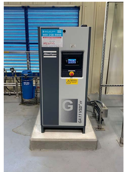
Duty and standby compressors charge the receiver tank which supplies compressed air to the valve module.
