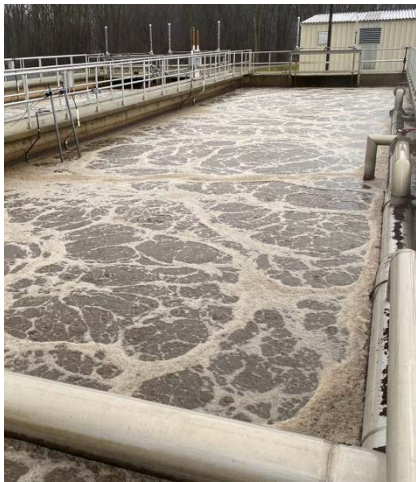
Ground level view of aeration train
