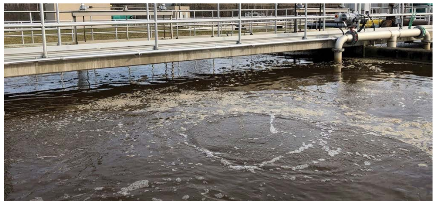
BioMix Compressed Gas Mixing in operation
