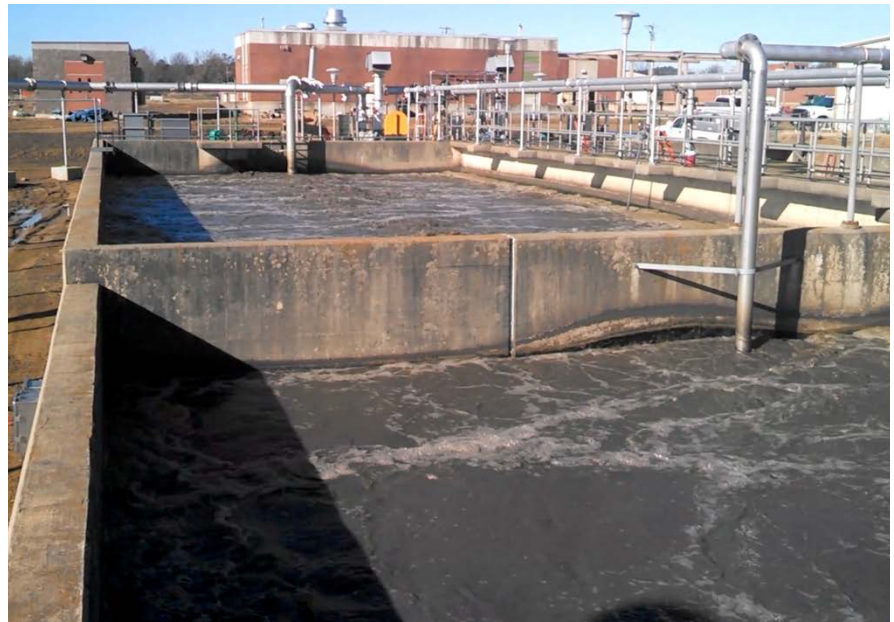
The Russellville PCW facility
